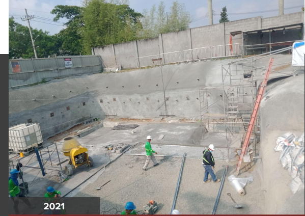
Westborough Cistern Tank (Silang, Cavite) - 2021
